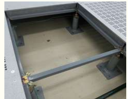
Raised Panel Flooring
